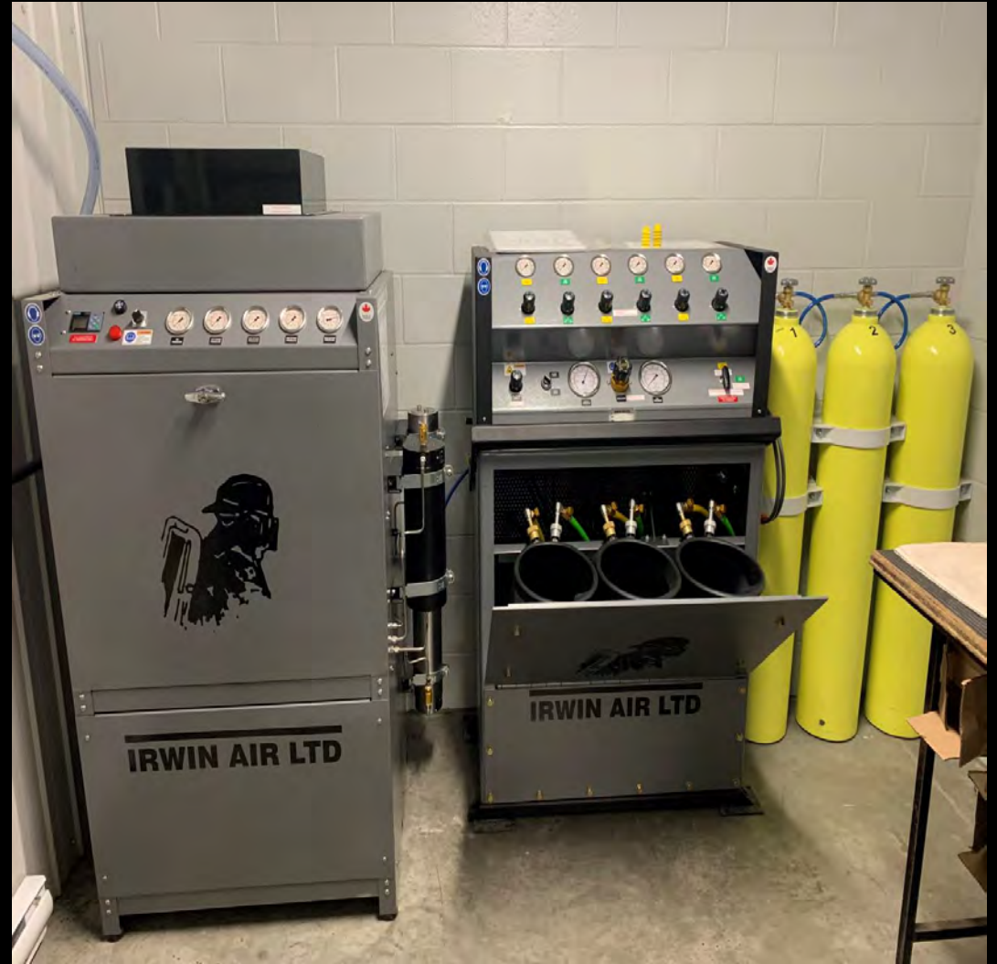
Breathing Air Compressor and Fill Station
